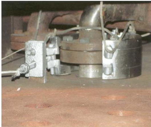
Fig. 6 Clamp fixed around leaky flange
