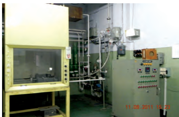
Fig. 5. PCF at Dhruva reactor
