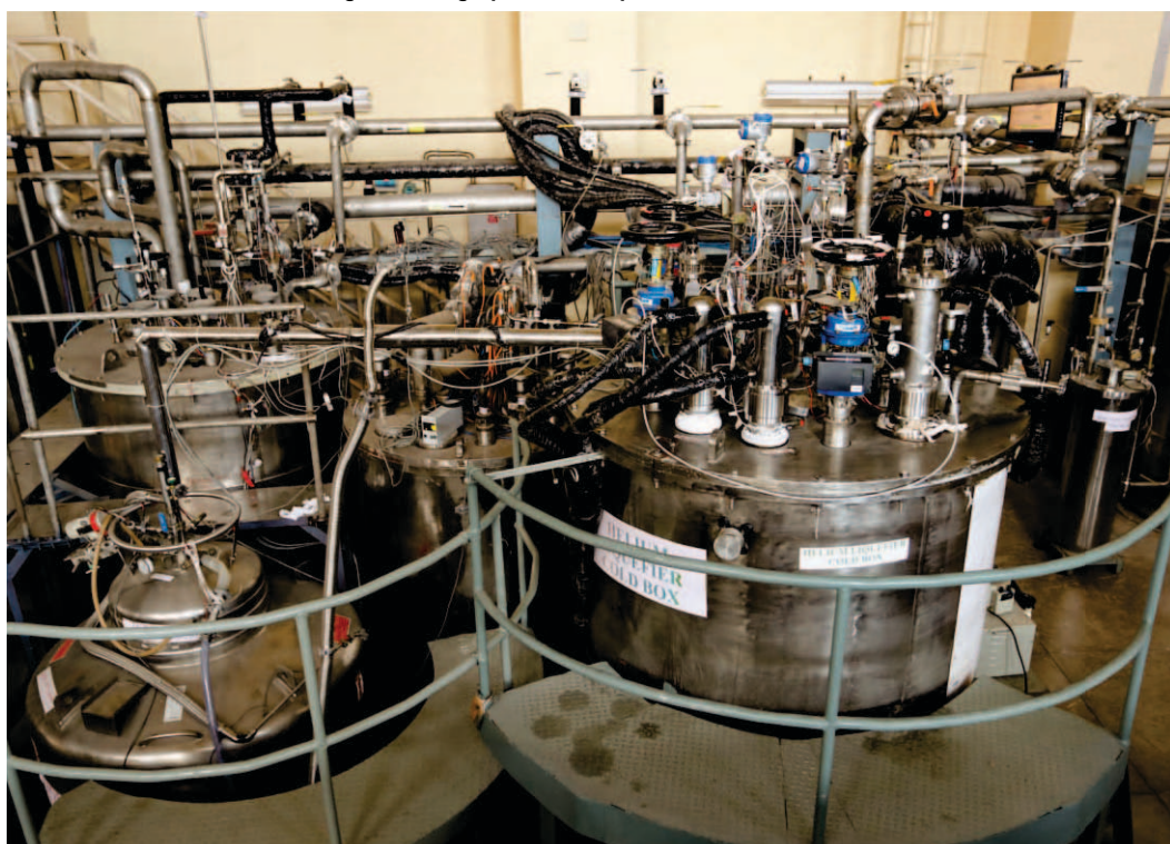
Fig.6: Developed helium refrigeration/ liquefaction system
