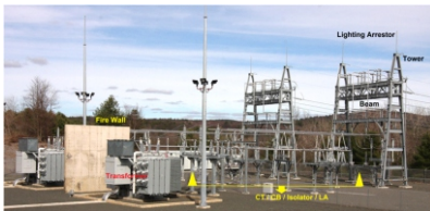
Typical Electrical Substation of a Nuclear Facility
