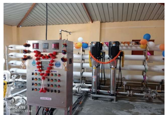
12500 LPH capacity water treatment unit (Inside view)
