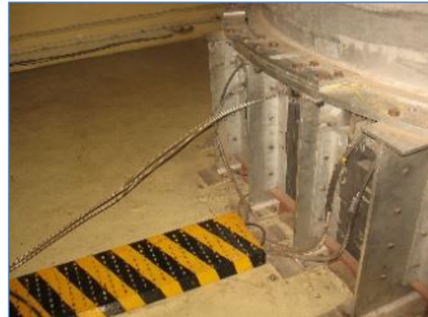
Signal cables coming out in the Reactor Pit
