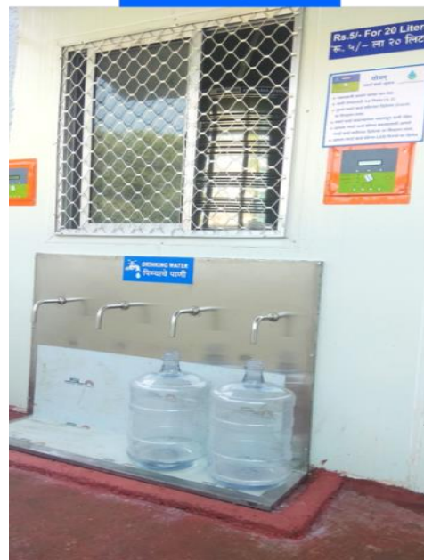
Water ATM facility of 1000 LPH RO plant at Somthana, Maharashtra.
