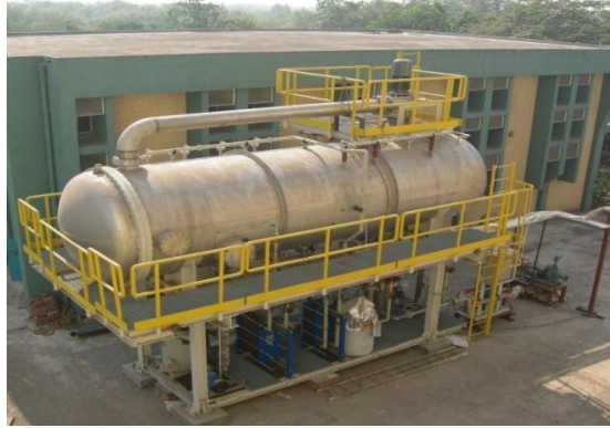
50000 l/d MED-MVC Plant at BARC, Trombay
