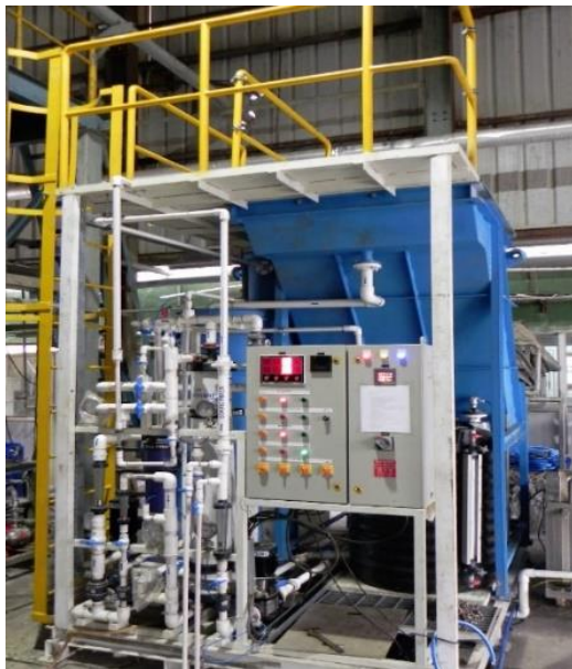
Brine Purification Unit
