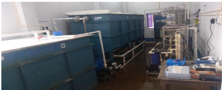
1000 LPH As removal plant set up at Ichapur
