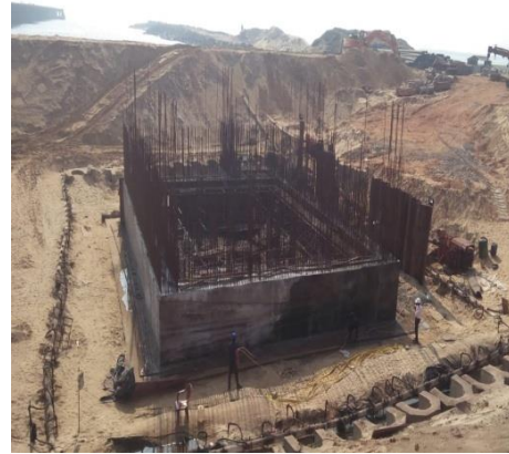
Sea Water intake pump house
