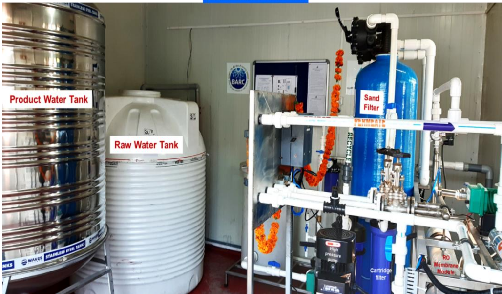
Inside view of 1000 LPH RO plant installed at Somthana, Nanded, Maharashtra.
