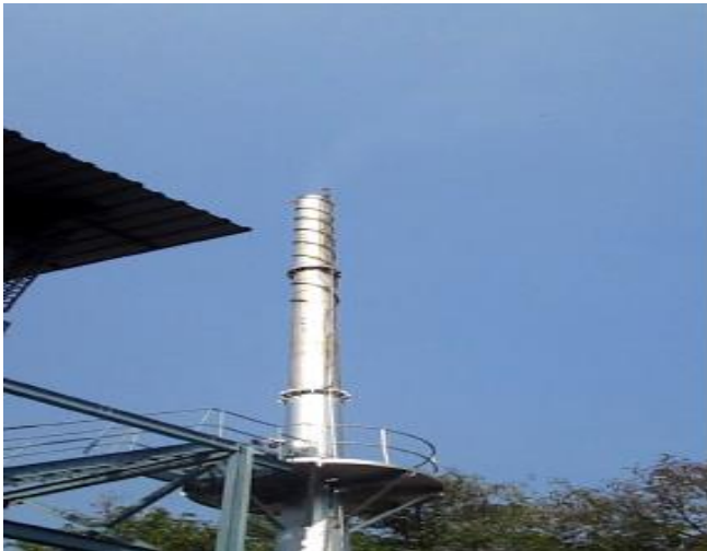
Clean emission from stack: Only faint white stream of water vapour
