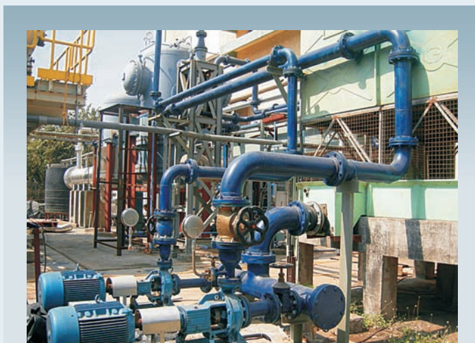
Next Generation LTE-CT Plant at Trombay (50 KLD capacity)
