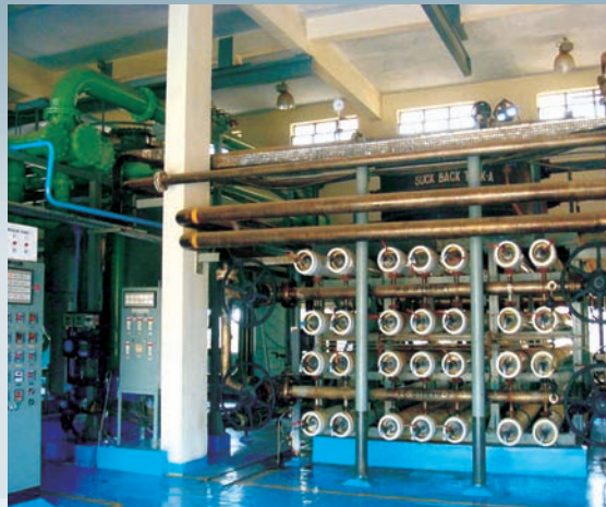
1.8 MLD SWRO Plant at Kalpakkam
