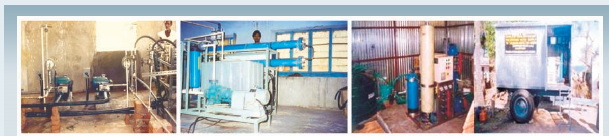
Brackish Water Desalination Plants in Rural Areas (5-30 KLD capacity)
