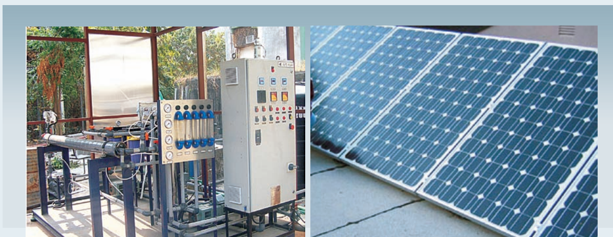
Community Level RO Plant along with PV Panels (250 LPH)
