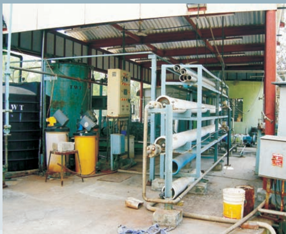
100 KLD SWRO Plant at Trombay
